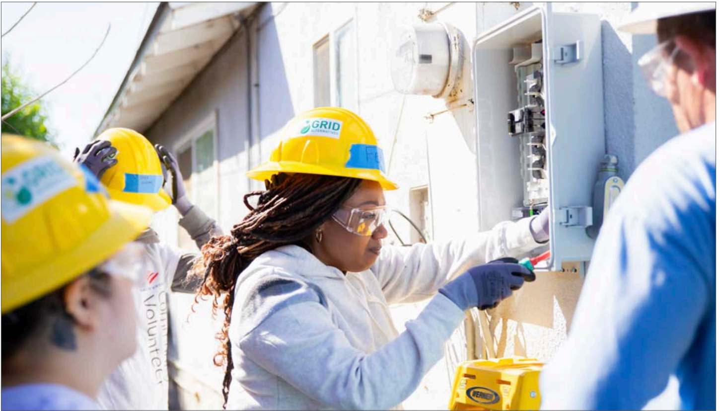
GRID Alternatives trainees upgrading an electrical box to accommodate rooftop solar panels. Photo credit: GRID Alternatives
