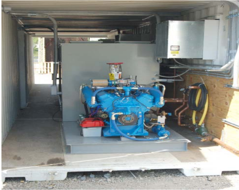
Figure 3. Tecogen Prime Mover with Inverter
