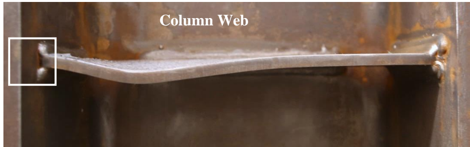
(a) East Bottom Flange Continuity Plate
