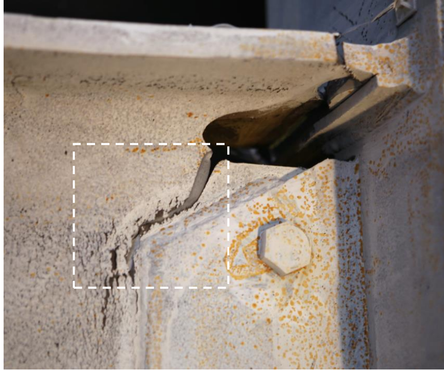
Figure 4.174 Specimen W4: East Beam Top Flange Weld Access Hole Fracture during First of - 0.05 rad
