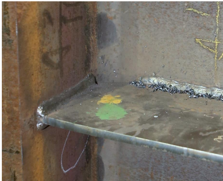
Figure 3.16 Continuity Plate Fillet Welds (Specimen C5)
