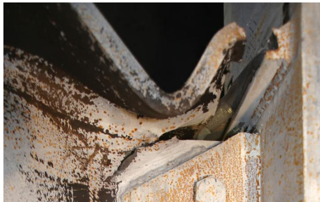
Figure 4.149 Specimen W3: East Beam Top Flange Weld Access Hole Tear
