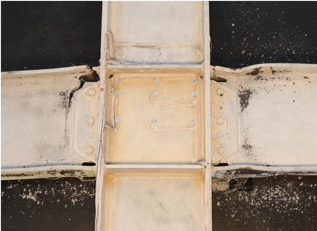
Figure 4.177 Specimen W4: Connection at End of Testing
