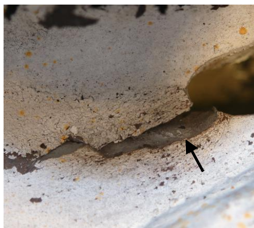
(b) Weld Fracture
