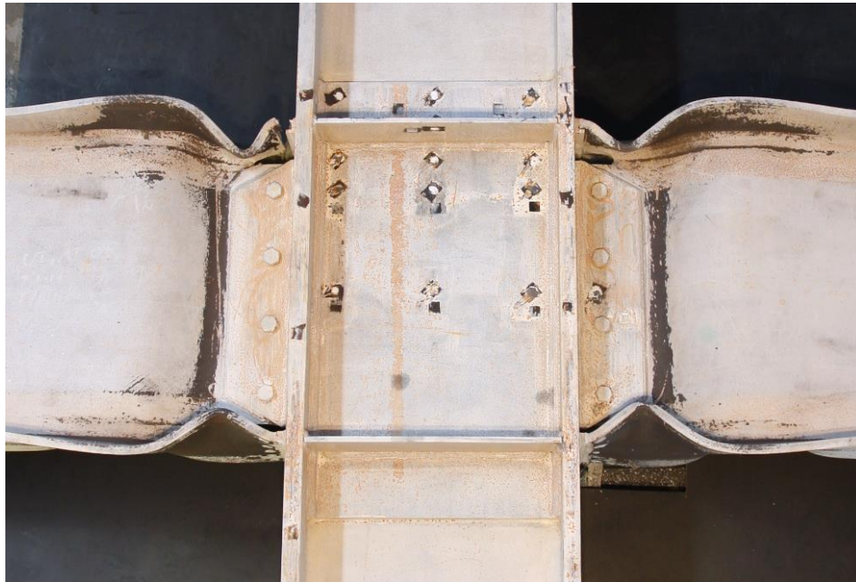
Figure 4.152 Specimen W3: Connection at End of Test
