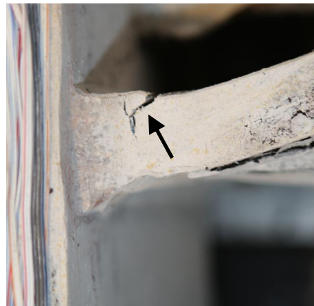
(b) Weld Fracture
