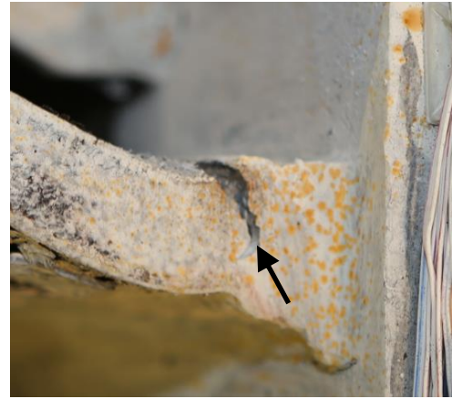
(b) Weld Fracture
