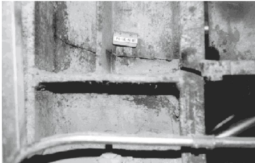
Figure 1.2 Fracture at Beam Bottom Flange Steel Backing Bar (Hamburger et al. 2016)
