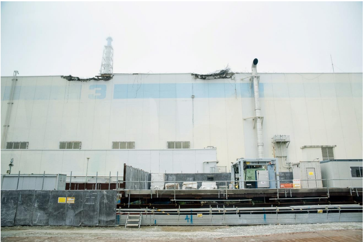
Figure 80: Nuclear reactor #3 shows building damage (7/11/2016)
