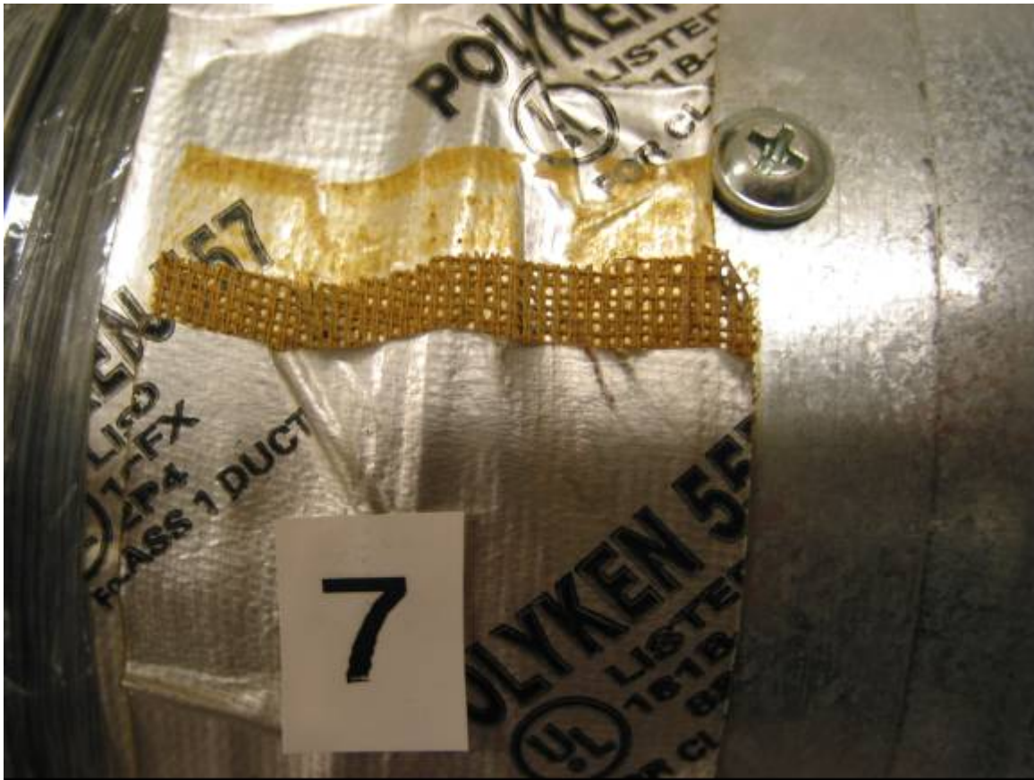
Figure A7. Sample 7. Like sample 6, sample 7 shows considerable shrinkage and delamination.
