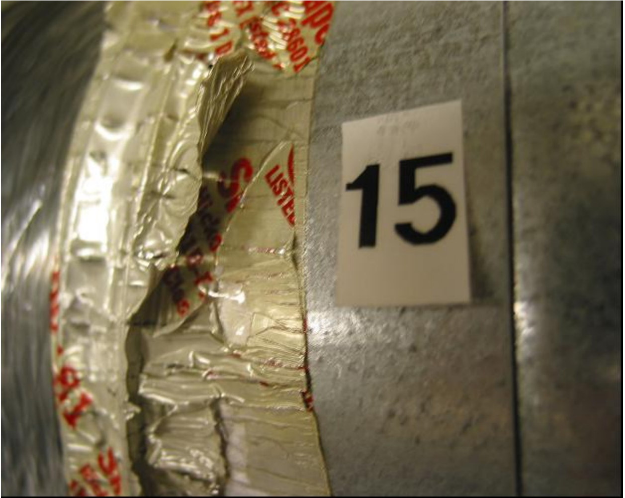
Figure A18. Sample 15. Like samples 13 and 14, this sample is also peeling and cracking. This figure shows how the metallized layer is splitting from the adhesive layer.
