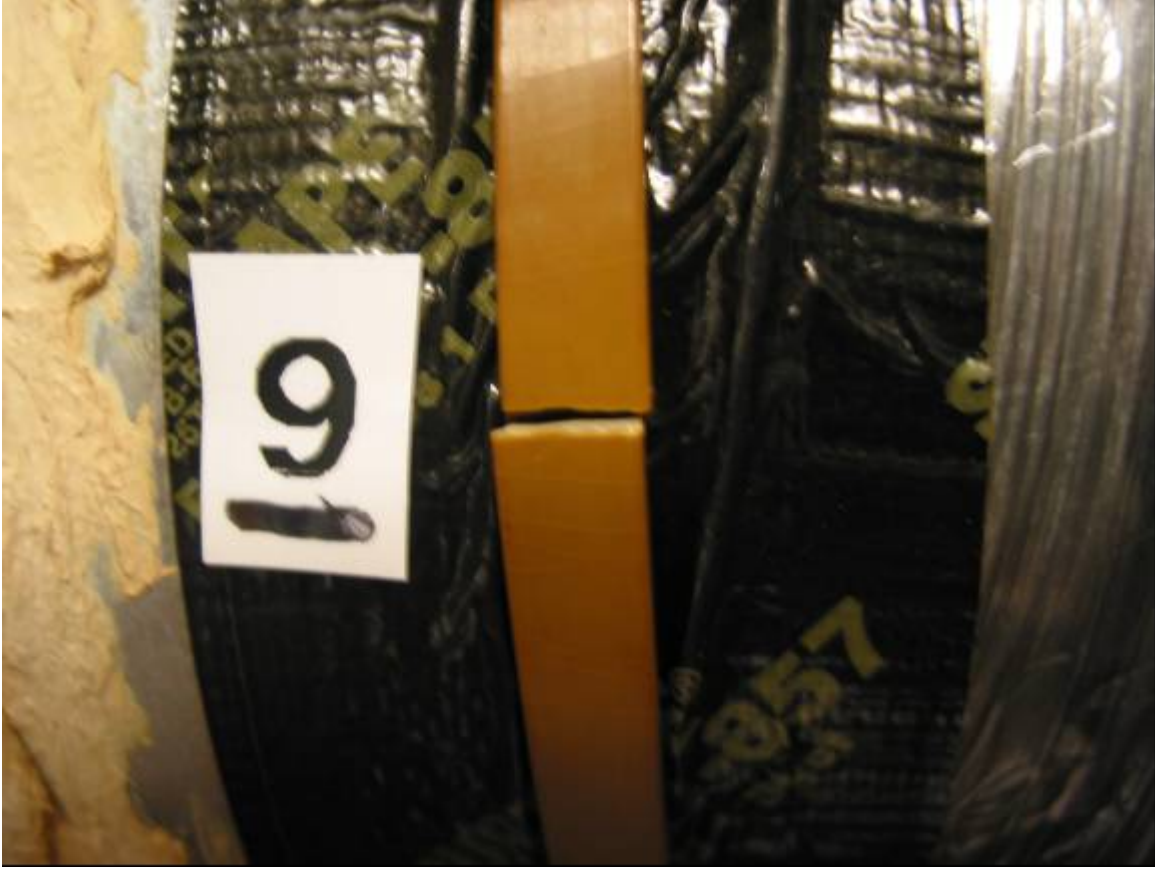
Figure A10. Sample 9. The clamp shows its brittle failure. Note that these clamp sections are now held in place because they are stuck to the duct tape.
