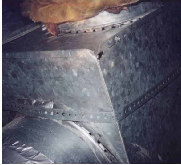
Figure 1 Example Of Collar-To-Plenum Connections On A System Where The Tape Sealant Has Fallen Off
