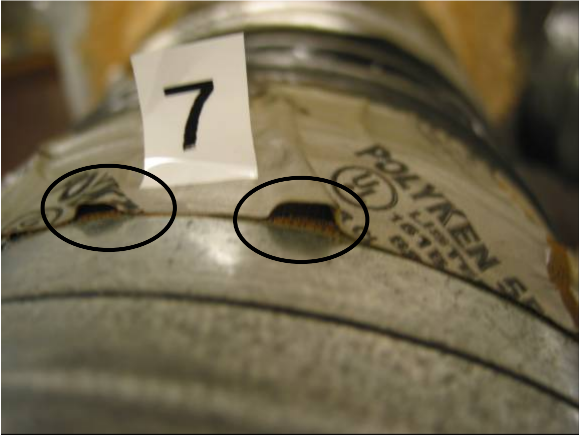
Figure A8. Sample 7. The edges of the tape have lifted off the duct surface in large wrinkles.
