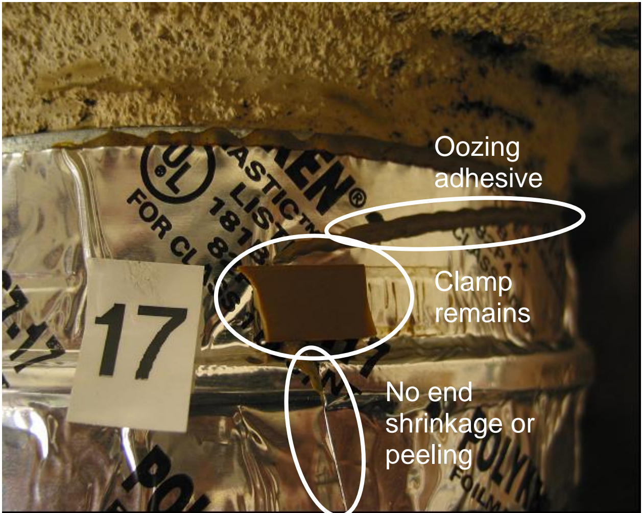
Figure A20. Sample 17. As with sample 16, this metal foil tape is showing oozing of the adhesive. Note that there is no shrinkage or delamination like the other tapes at the end of the tape. There is also a small piece of clamp stuck in place by the oozed adhesive.
