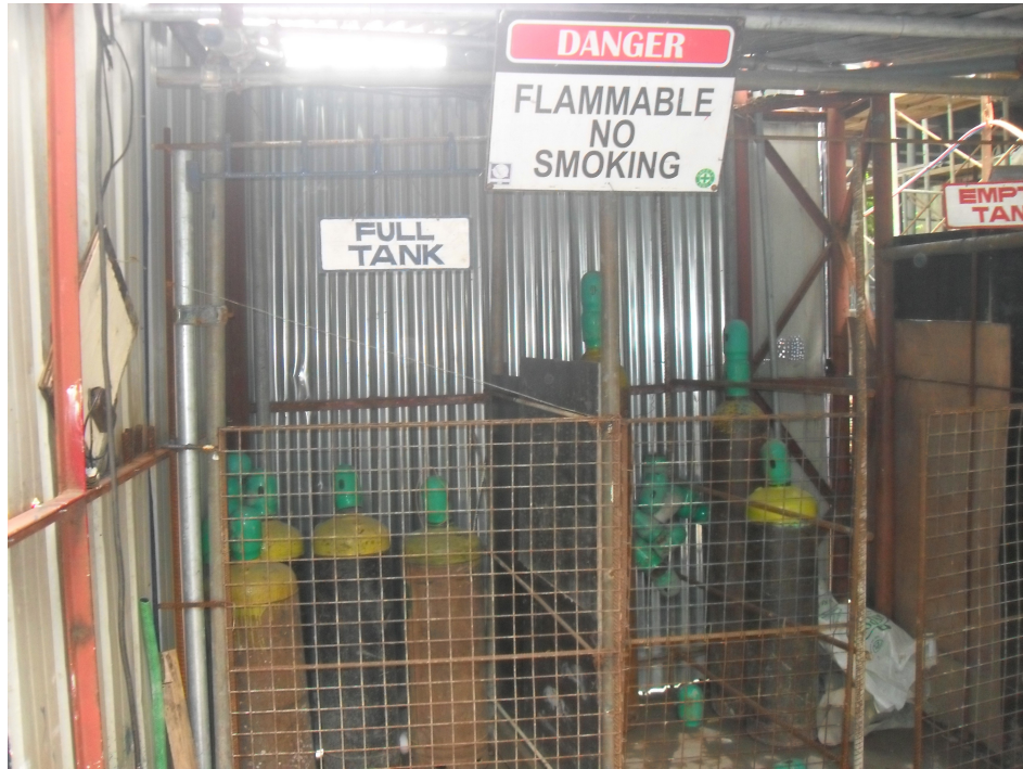
Figure 16: Proper Storage of Fuel tank
