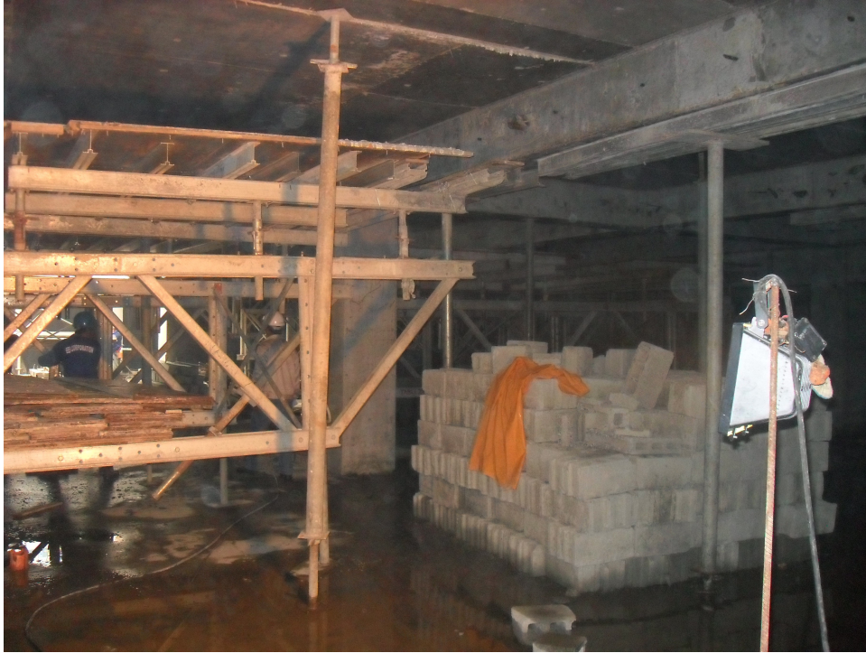
Figure 14: Proper & Adequate Lighting
