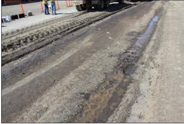
Figure 3.19: FDR-EE: Puddled water on surface after compaction.
