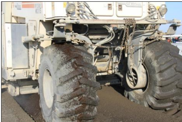
Figure 3.16: FDR-EE: Excess emulsion applied during recycling.
