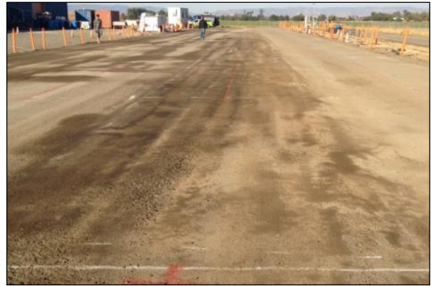
Figure 3.35: Broomed surface of FDR-EE layer showing dark, moist surface.
