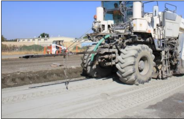
Figure 3.27: FDR-PC: Excess cement on Cell #7.
