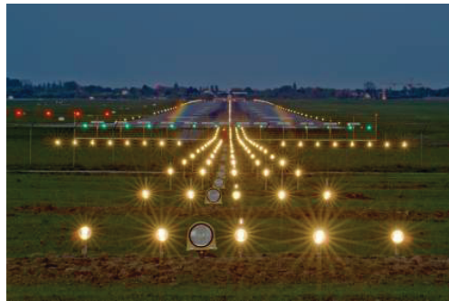
Figure 2.3: Airport LED guiding lights.
