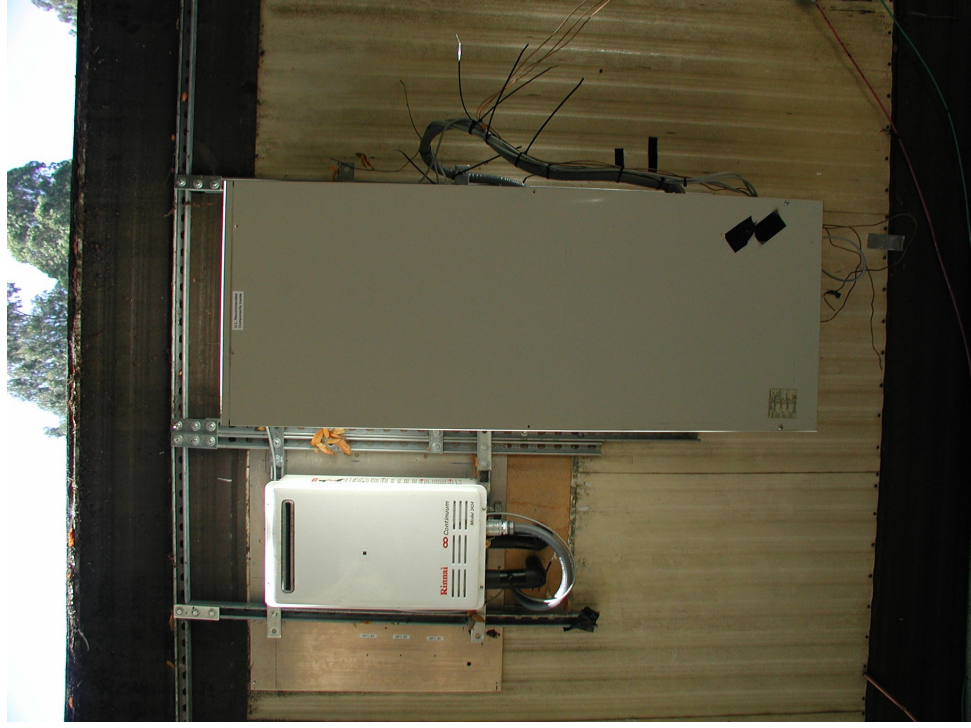
Figure B1. IDEC and instantaneous hydronic heater mounted on B67C wall.
