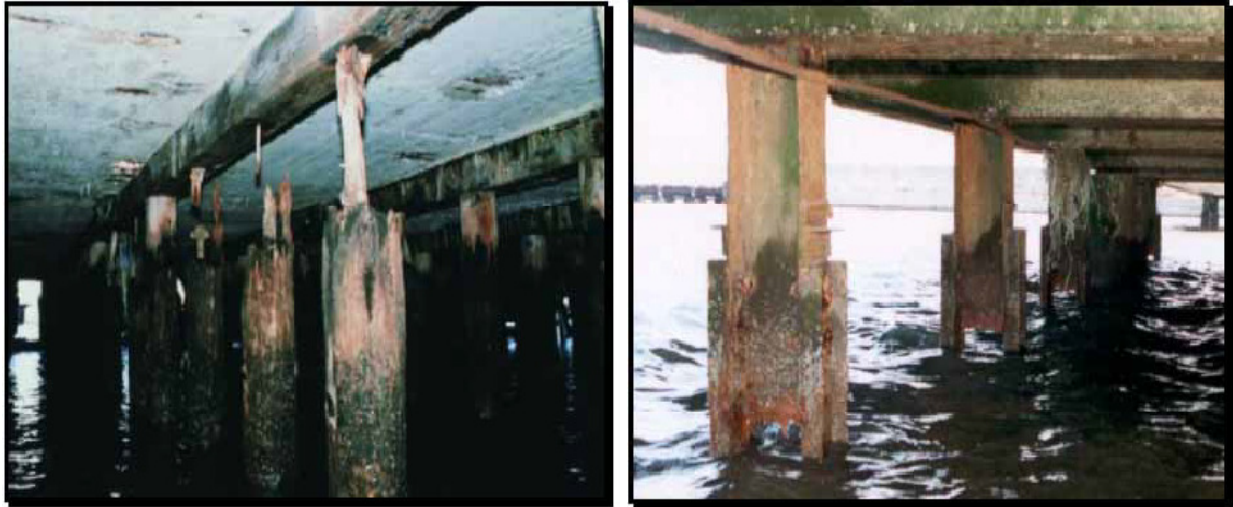
Figure (1.1): Deterioration of conventional timber and concrete piles
