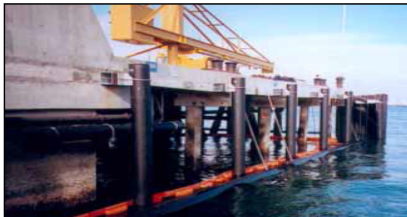
Figure (1.2): Fender piles in the U.S. Naval Submarine Base, San Diego, CA
