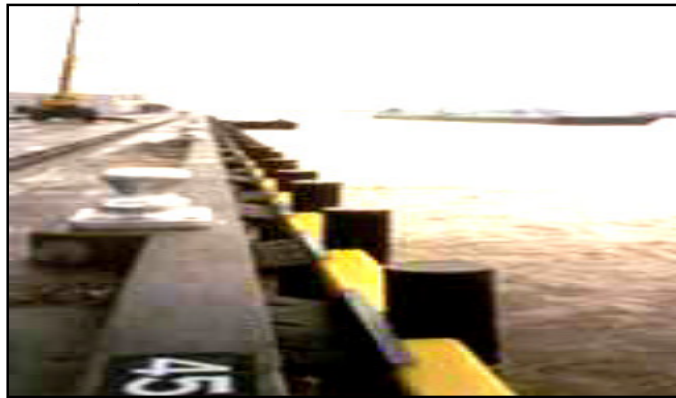
Figure (1.4): Fendering system, Nashville Avenue Marine Terminal Port of New Orleans, LA, USA
