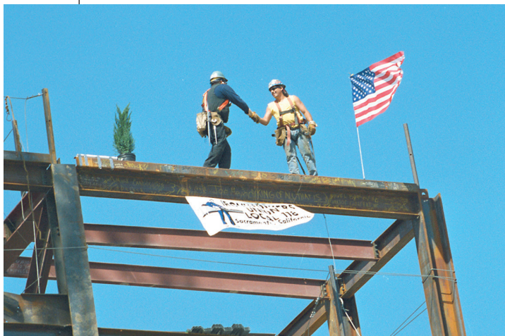
Two construction workers shake hands at the March 2001 “topping out” ceremony celebrating the placement of the center’s last steel beam. (Photo: UC Davis)
