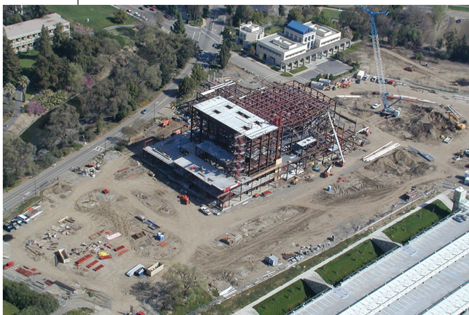
The center's soaring steel frame rises from the ground in March 2001, anchoring the campus's new south entry and sitting kitty-corner to the Buehler Alumni and Visitors Center. (Photo: D. Kern Holoman/UC Davis)
