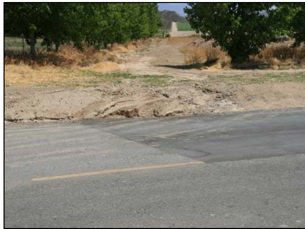
Figure 2.8: Access road drainage problems (note digout).
