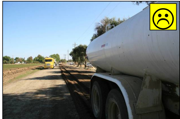
Figure 6.40: Primary compactor too far behind recycling train.
