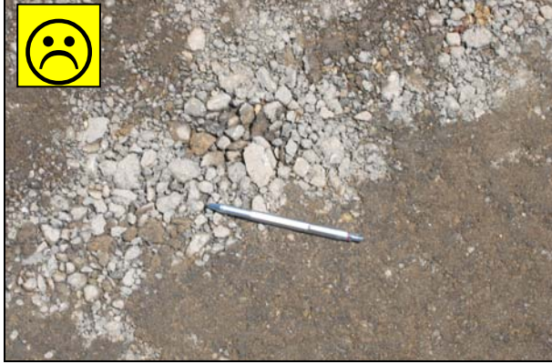
Figure 6.44: Segregation after grading.
