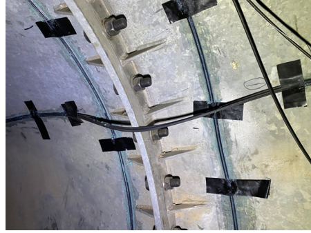
(b) Close-up of fiber optic cables jumping the flange and the stiffeners at the flanges.
