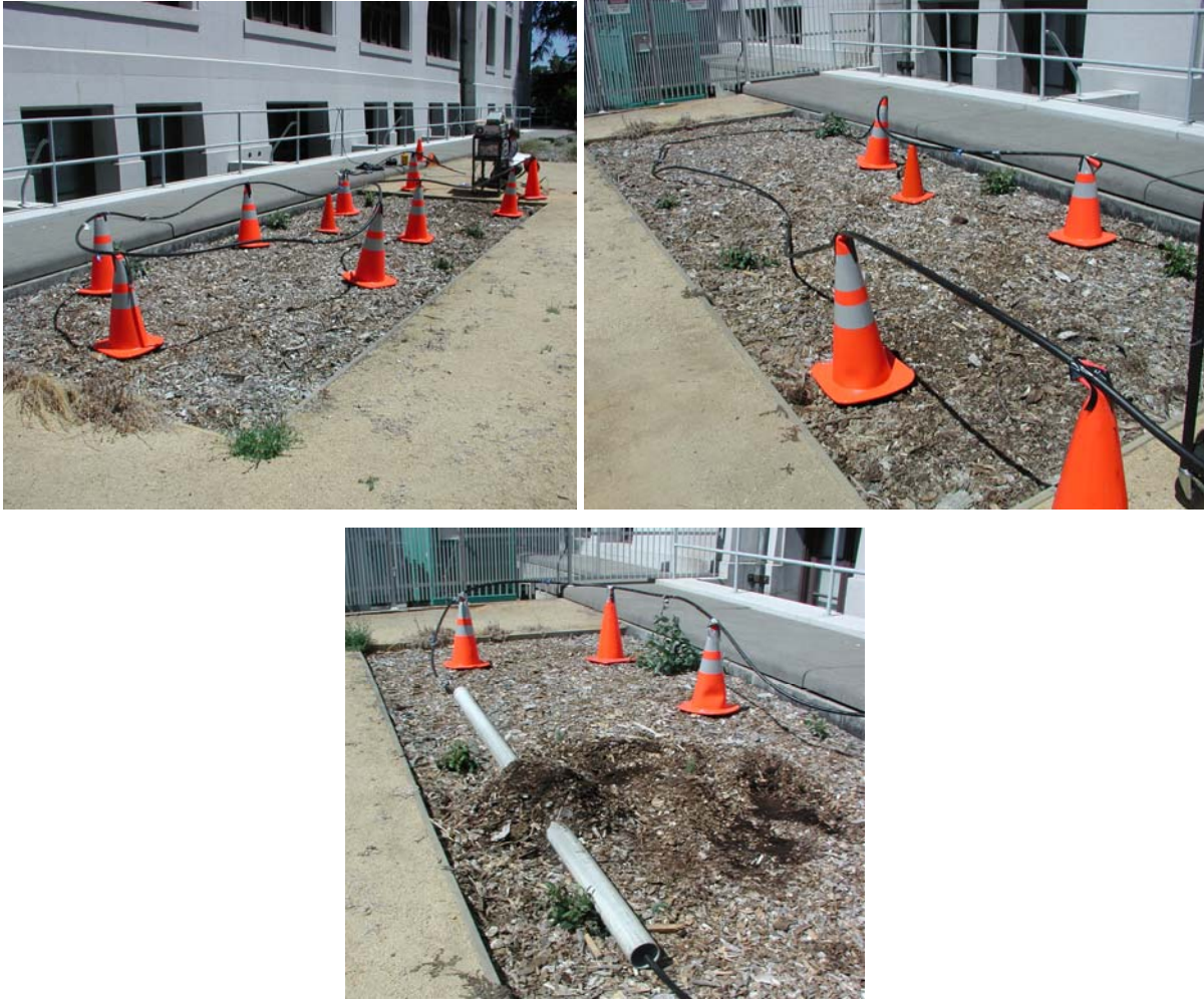
Figure 3. The 64 feet outdoor underground cable GW setup. The cable was at times completely ( top-left ) or partially ( top-right, bottom ) supported by 29-inch tall plastic traffic cones.
