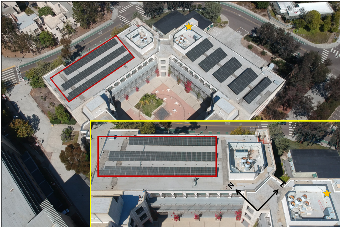
Figure 4.2: Aerial view of the PV system installed on EBU2 at UCSD and the PV production field (red) considered in this paper. The yellow star indicates the CSS located 10 meters north of the upper corner of the PV system. ©Drone Photo
