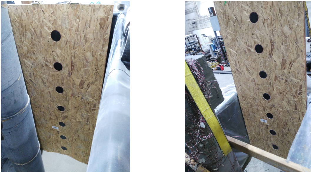
(a) Original soil pressure sensors' disposition. (b) Soil pressure sensors on top of the bedrock.
