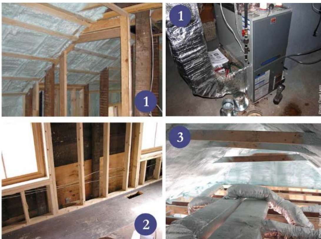
Figure 7 Images from Belchertown DER (clockwise from top left), including sealed and insulated attic, high efficiency forced air gas furnace, new stud wall built to interior of old structure, and HVAC ducting insulated and in conditioned space. Images courtesy of the Building Science Corporation.
