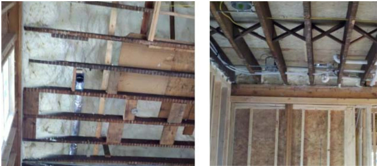
Figure 10 Left : unvented attic sealed with closed cell spray foam. Right : insulated band-joint. Images courtesy of Oak Ridge National Lab.
