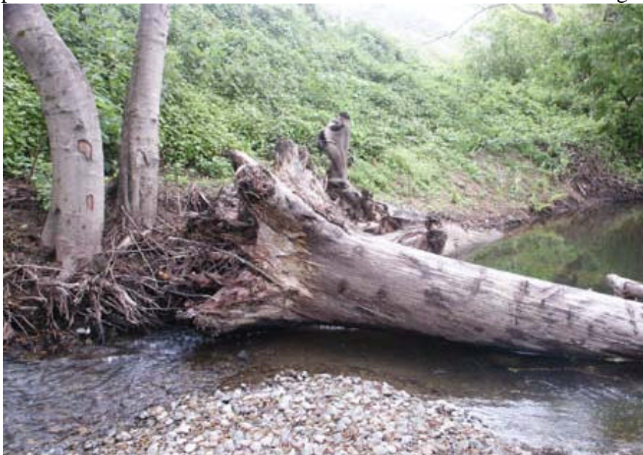
Photo 14. Exposed tree roots on left bank near weir structure 6-7-8. Bar 6 in foreground.
