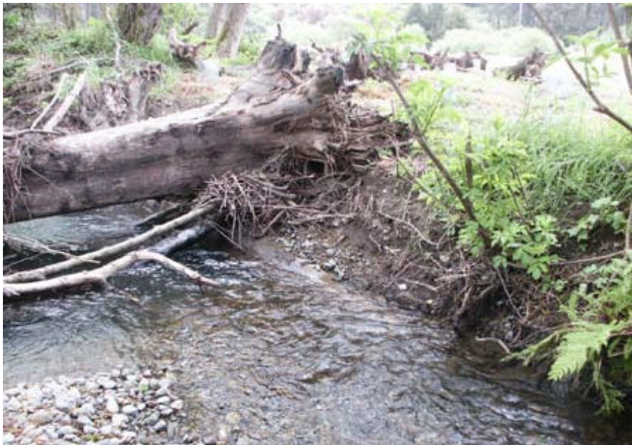
Photo 12. Exposed tree roots and eroding bank area on right bank upstream of weir structure 6-7-8.
