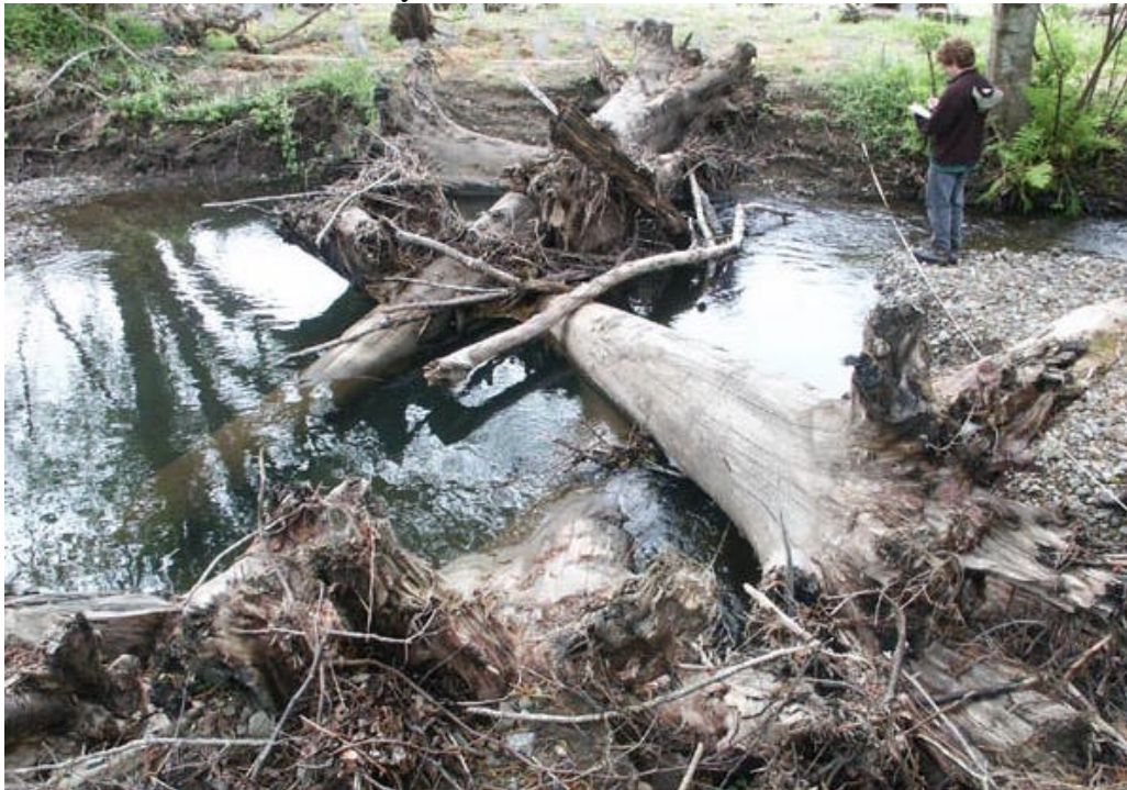
Photo 4. Looking towards the right back at weir structures 6, 7, and 8. A pool has scoured directly downstream of the structure.
