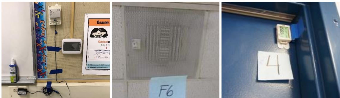
Figure 1. Sensors deployed in schools to measure room CO 2 , air temperature and RH (left), supply air temperature and relative humidity (middle), and door open/close state (right).
