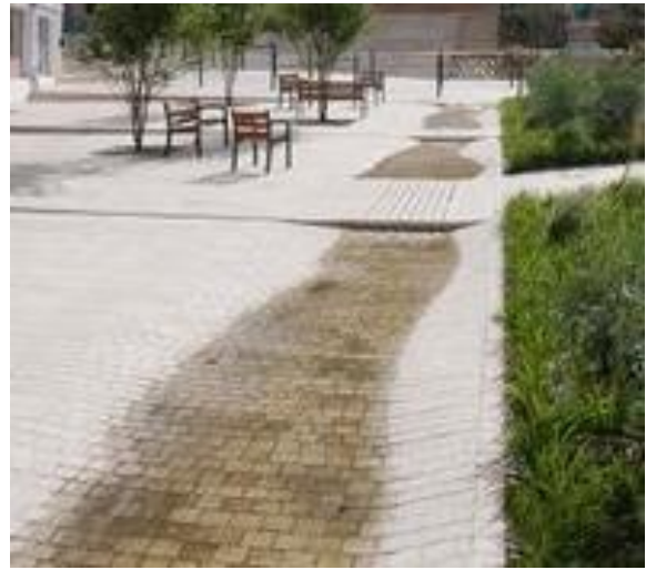
Figure 13.81 The pavement transformed into a water channel in Gondrecourt-le-Chateau (Picture source: https://www.pinterest.com/ezrarem/rills-and-runnels/ , retrieved January 22, 2016)
