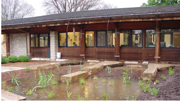
Figure 13.146 The scuppers of the International Student Center at Kansas State University (Picture source: http://artfulrainwaterdesign.psu.edu/project/kansas-state-international-student-center-rain-garden , retrieved January 22, 2016)
