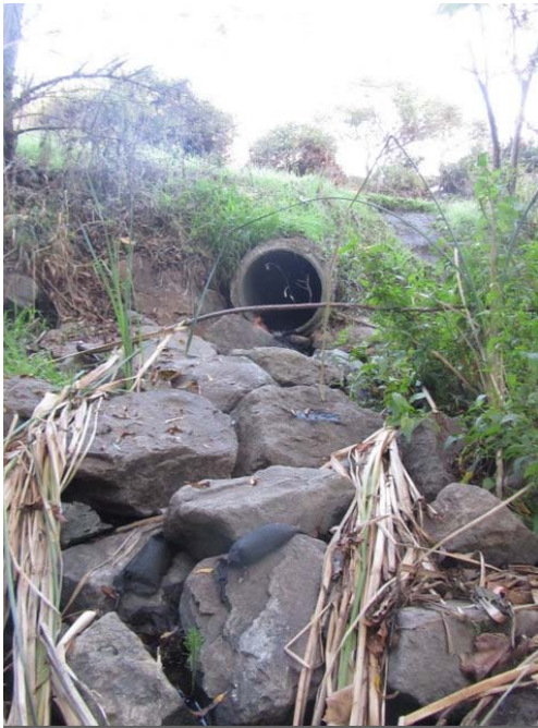
Figure B2: Stormwater outfall from El Cerrito Plaza parking lot to Cerrito Creek.
