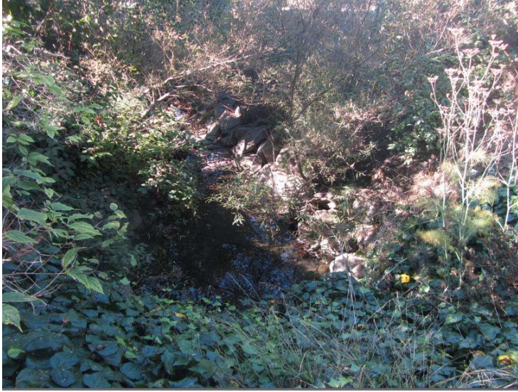
Figure B5: Deep pool just downstream of Talbot Avenue culvert. Invasive species as well as native plants are visible.
