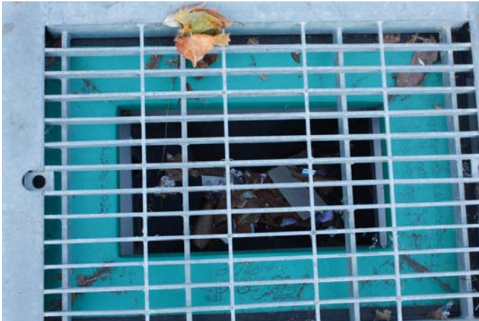
Figure B6: View into a parking lot drainage basin showing collection of debris and rubbish. Scheduled maintenance for these structures was undetermined.
