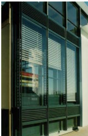
Exterior view (upper photo) and full-scale mock-up of the façade (lower photo).
