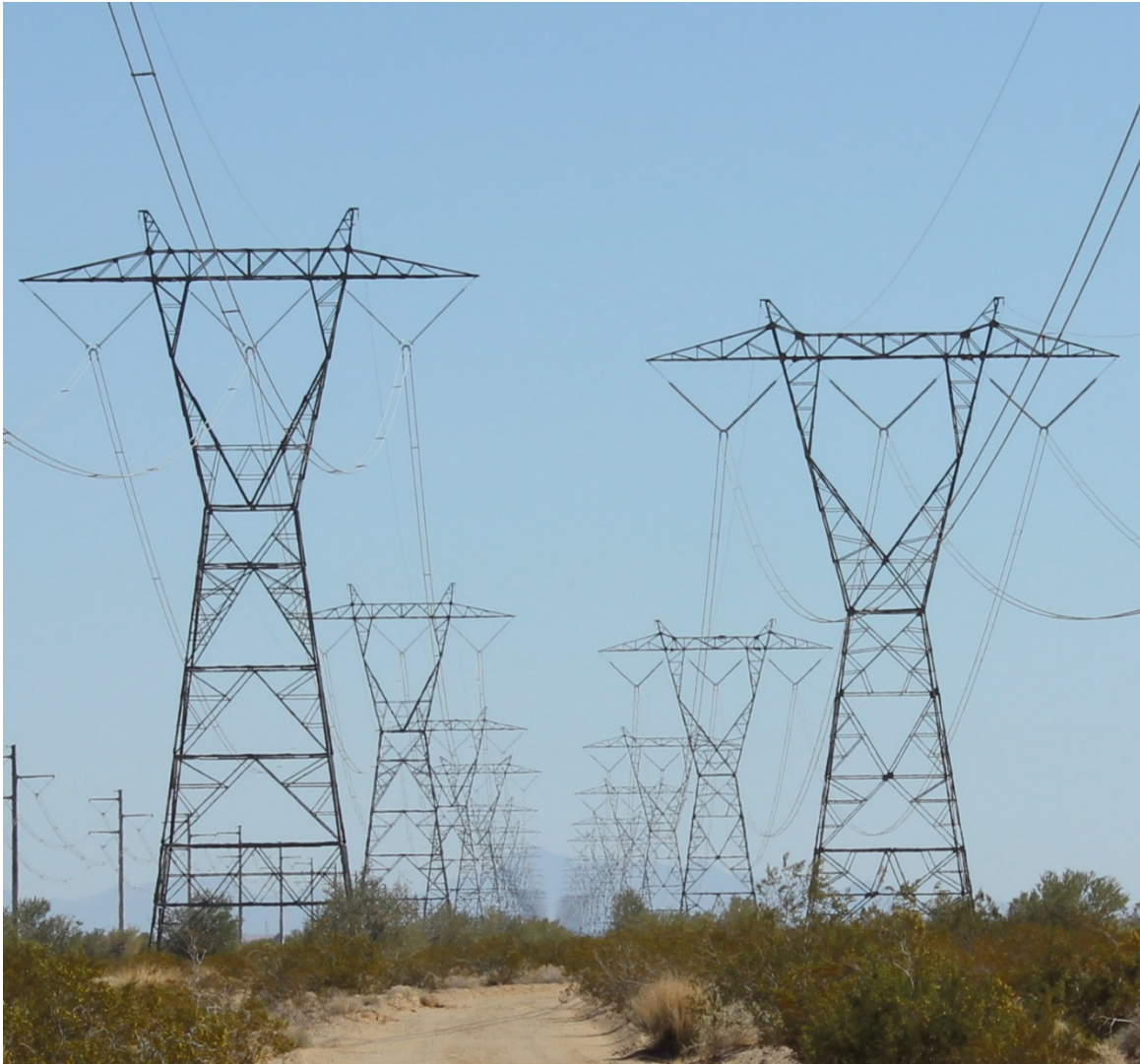
Figure 4-1. Lattice steel transmission towers in the lower Colorado Desert. Devers-Colorado River No. 2 (DCR2) is on the left in the image and Devers-Colorado No. 1 (DCR1) is on the right.
