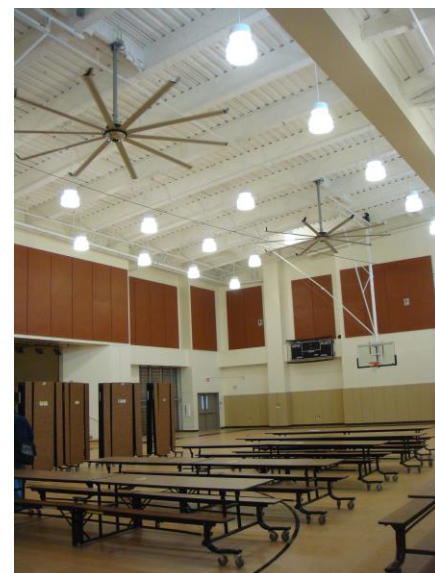
BSF ceiling fans in multi-purpose room
