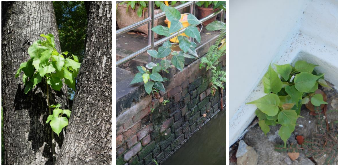
Figure 5: Pho kee nok. Bodhi trees that naturally grow by bird drops. They usually sprout from the cracks of old architecture which could cause damages to the structures. The senior monks said we must remove them before they grow too big. If they grow too big it will be difficult to cut both physical and psychological. People do not think there are tree spirits in small trees or even there are tree spirits, they would not be a strong or sacred ones.
