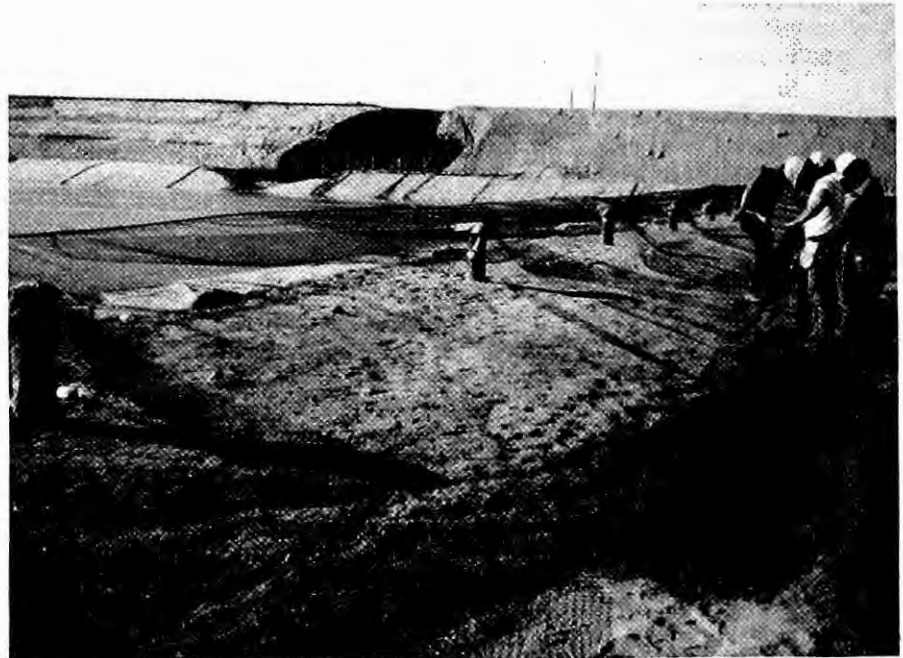
Figure 1. Support cables attached to pipes embedded in concrete facilitates a tight cable stretch. Workmen overlap the net 6 in and hog-ring the edges at 6 in intervals.
