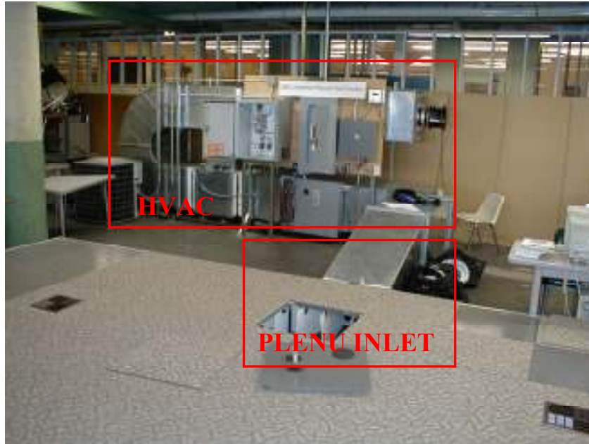
Figure 4-5 Plenum facility HVAC system and underfloor plenum
