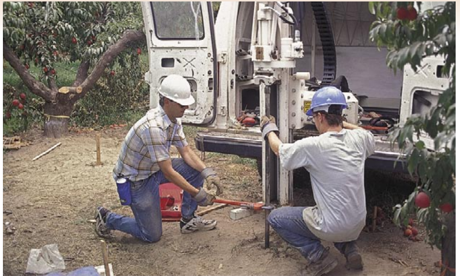
Nearly 3,000 feet of continuous soil cores were obtained between July and October 1997 using the Geoprobe direct-push drilling method. This method allowed for complete recovery of undisturbed cores throughout the 52-foot deep vadose zone. Above, UC Davis vadose zone hydrology professor Jan Hopmans (left) and Fresno State geology undergraduate Anthony Cole operate the coring equipment.
