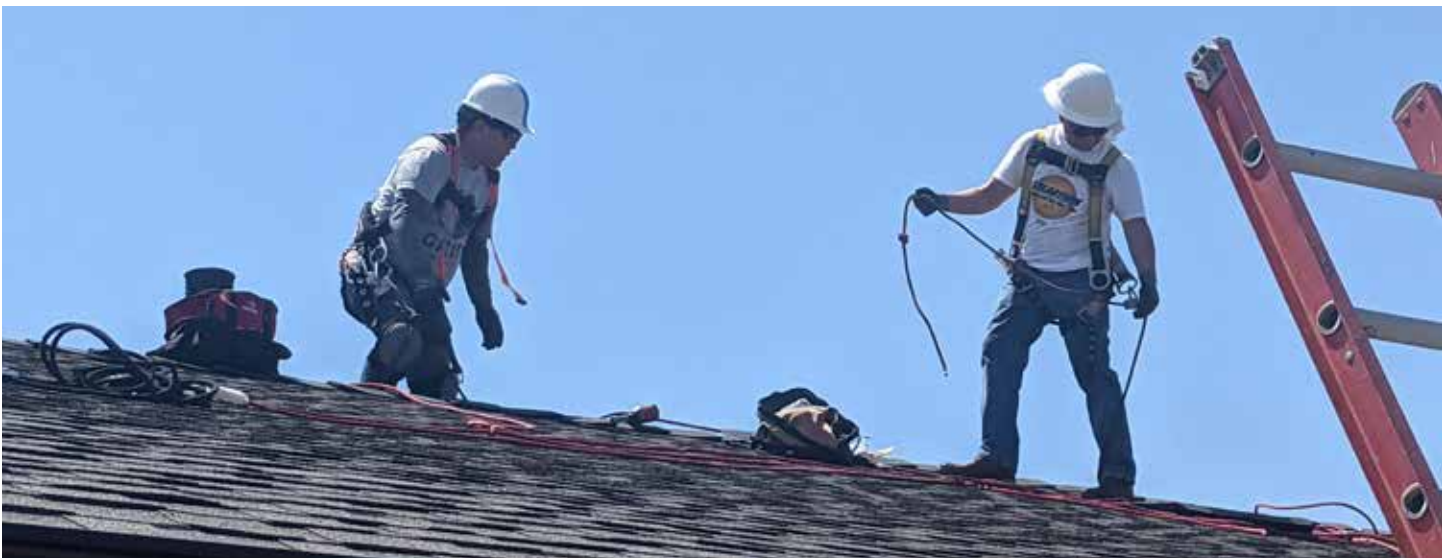
GRID Alternatives trainees installing solar panels at the first annual Solarthon event in June 2022. Photo credit: Pacoima Beautiful
