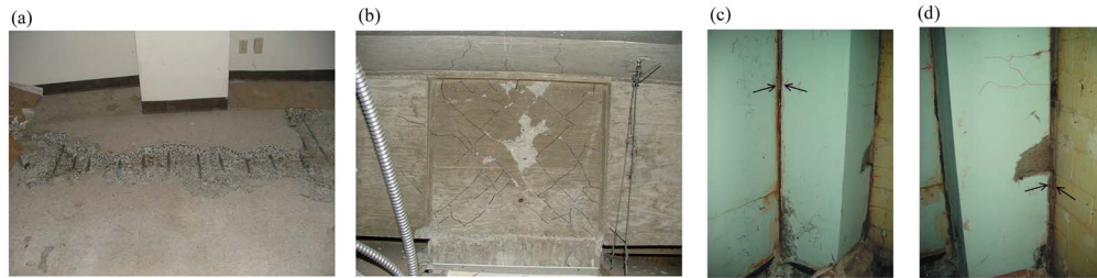
Figure 4. Earthquake damage to the building: (a) punching shear failure (Column B6 at the third floor level), and (b) diagonal crack on beam-column joint (Column A4 at the third floor level) (c) & (d) detachment of partition and infill wall from column (Column A1 at the first floor level).
