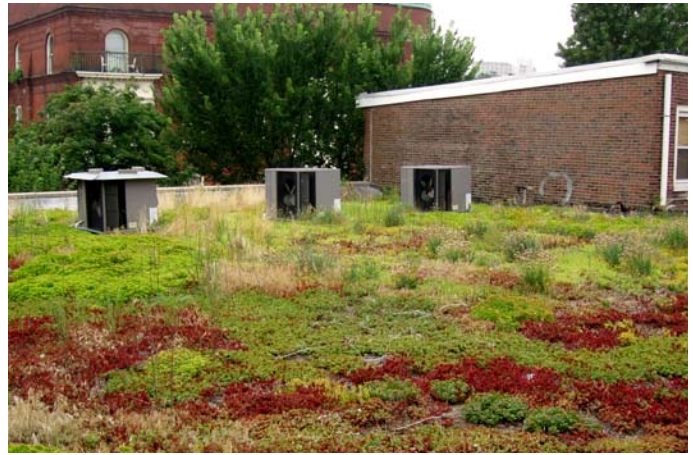
Figure 32. Green roofing installed to reduce runoff from a commercial building. Source: © Roofscapes, Inc., used by permission; all rights reserved.
