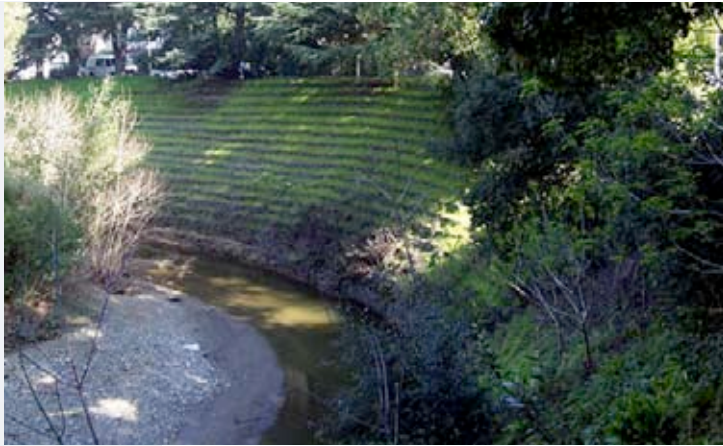
Figure 9. Gabion bank protection on San Francisquito Creek, Palo Alto, California, undertaken to stabilize the bank and reduce erosion. Photo: R. Harris.
