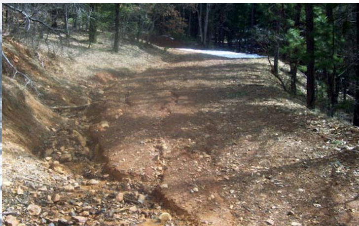
Figure 24. Erosion caused by ditch water leaving the ditch and traveling across the road. Photo: S. Kocher.
