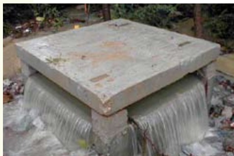
Figure 34. An outfall weir disperses storm water into a shallow area for infiltration. Photo: Deven Lindenberg, BLWI.
