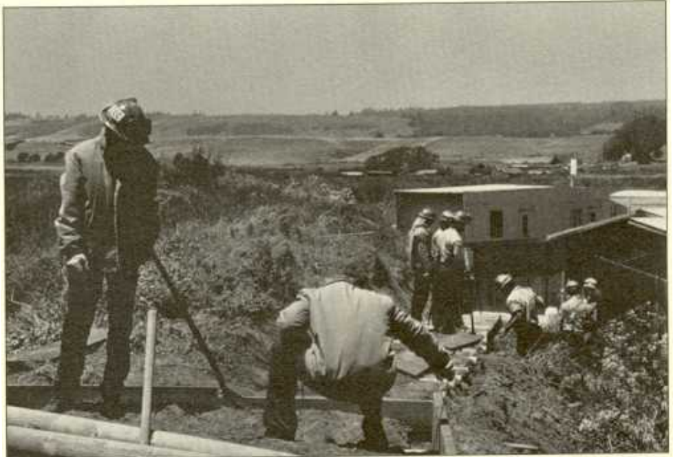
Hard-working Conservation Corps members needed just two weeks to construct a new beach overlook and 160-foot, handicap access trail at the Younger Lagoon Reserve. (Photo by Jim Keller)
