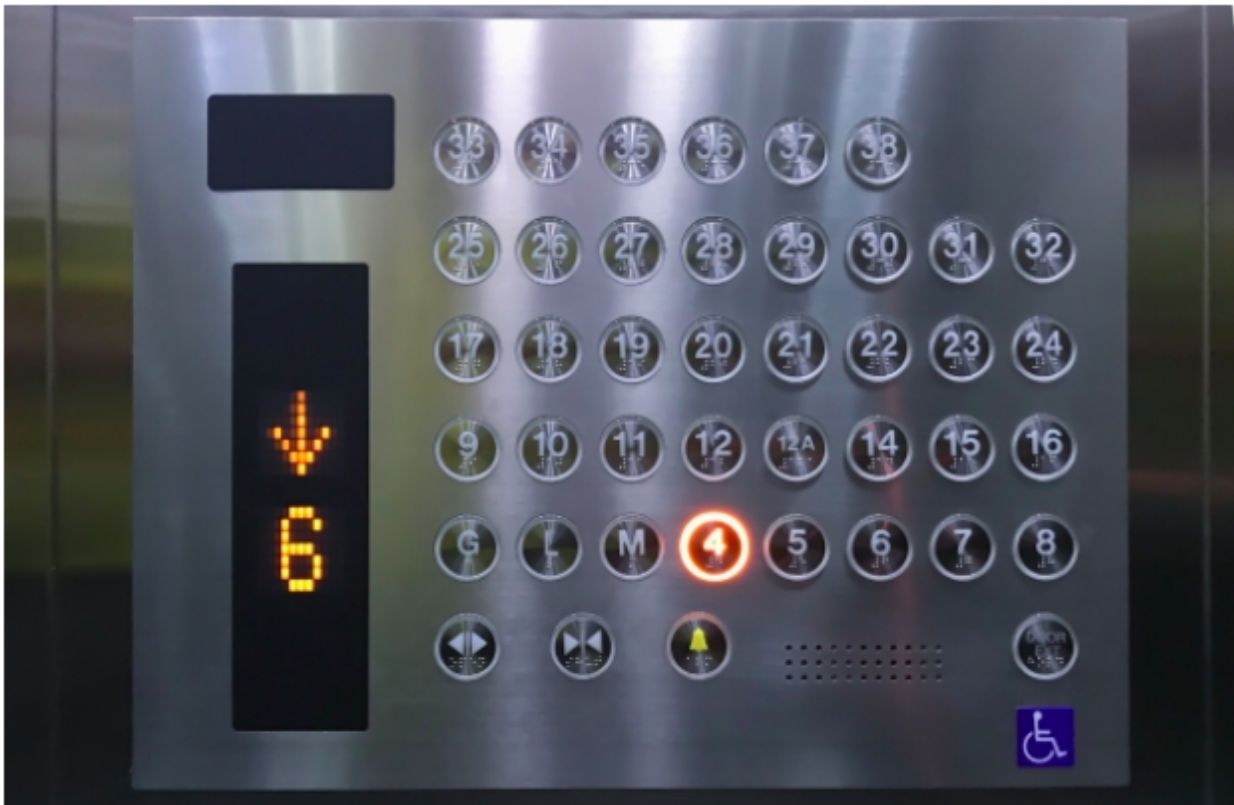
Figure 1. Elevator without 13th floor button
