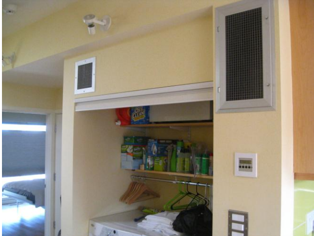
Figure 12 Failed HRV in Closet, Project 1201
