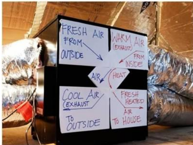
Figure 13 Airflow Labels on ERV, Project 1901
