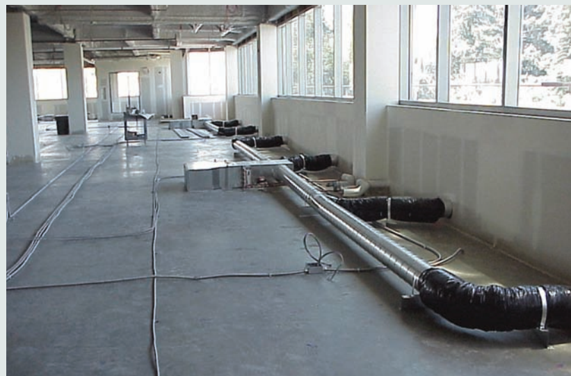
At the perimeter, underfloor variable speed fan-coil units are ducted to linear bar grille diffusers located on the window sills. These units draw supply air from the plenum as needed during cooling operation and provide heat from hot water coils during heating.
