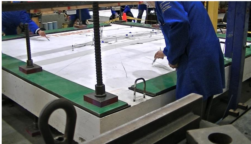
Figure (3.48): Cracks Initiation, Propagation and Size Growth were monitored throughout the Test
