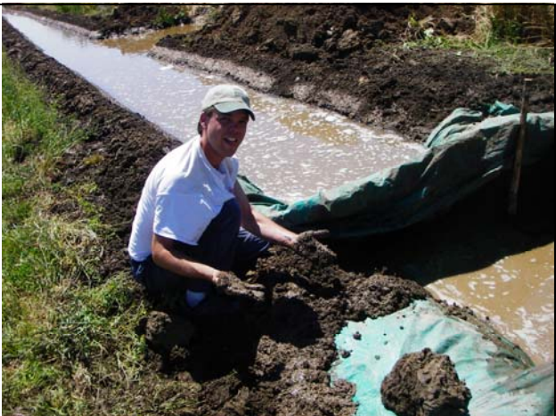
DO-101 WPF-UD-IN Jeremy Hanlon working on weir structure for inflow into un-vegetated ditch.
