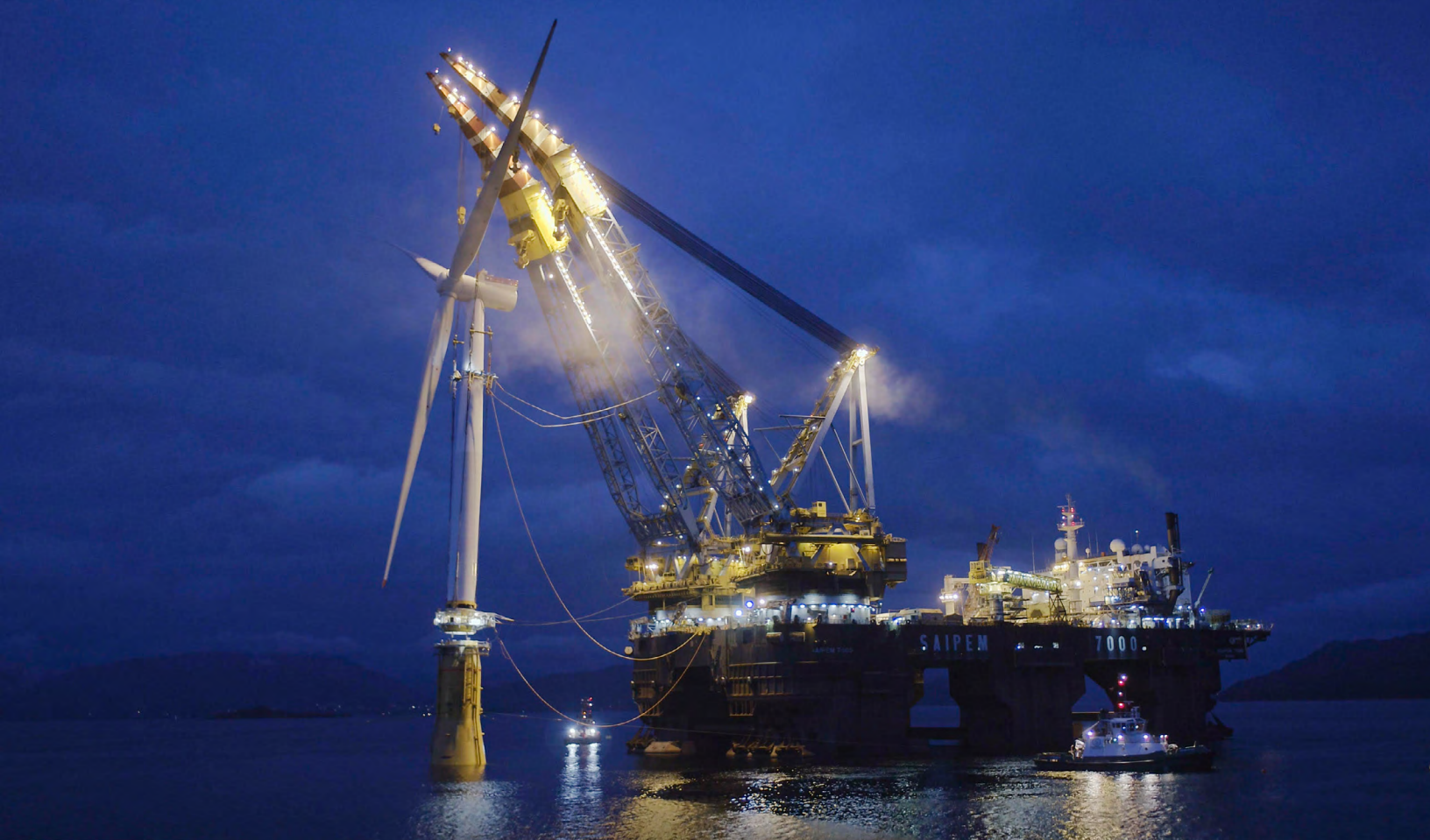
A turbine being “mated” with its underwater substructure prior to being installed at Hywind Scotland, the world’s first commercial floating offshore wind farm, which began operations in October 2017. Photo: Statoil
