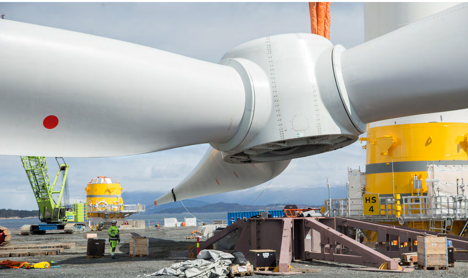
Turbine assembly at port in Norway prior to being towed to Hywind Scotland, the world's first floating offshore wind farm. Photo: Statoil
