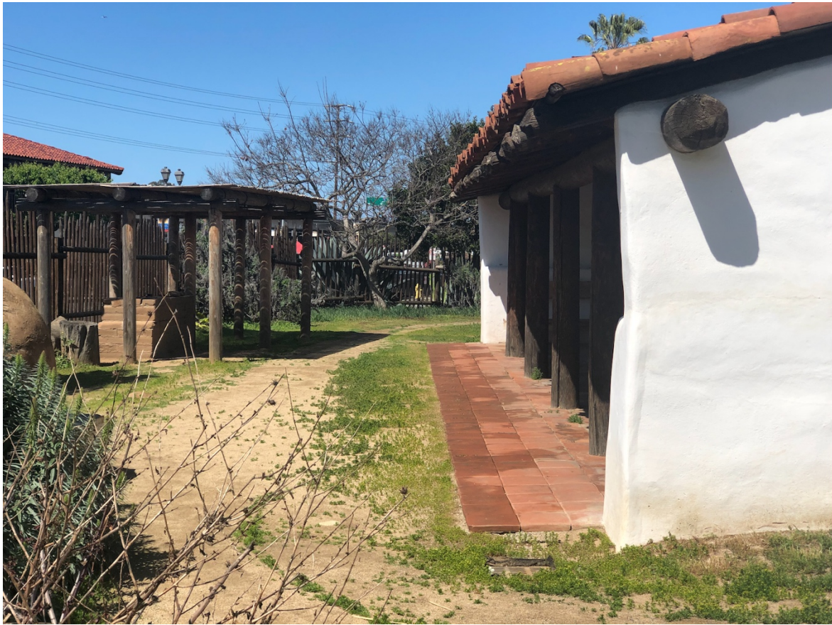
Figure 7.11: Rear exterior of the casa displaying the restored outdoor kitchen area featuring an open-air cooking capacity in the far left of the frame as well as outdoor seating (not visible) underneath the casa 's built-in pergola (right side), illustrating another aspect of domestic life. Photo by author, 2019.
