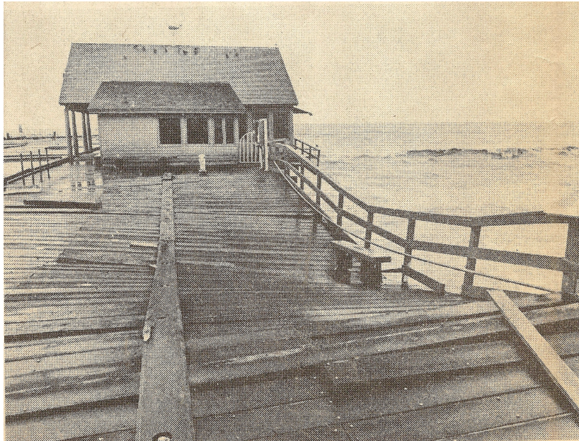
Figure 2.9 Large waves that arrived during high tide and an elevated sea level in March 1983 left Stearns Wharf sagging from a loss of pilings (source: Santa Barbara News-Press).
