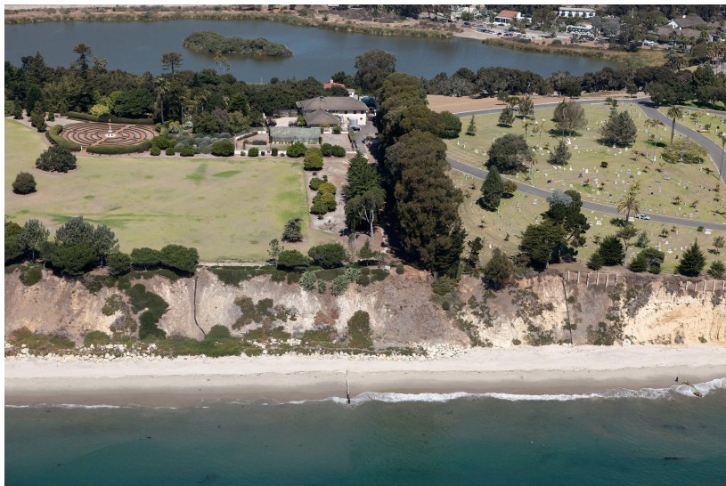
Figure 2.3 Cliffs are actively eroding along the Clarke Estate and the adjacent cemetery (photo: Kenneth and Gabrielle Adelman, California Coastal Records Project).
