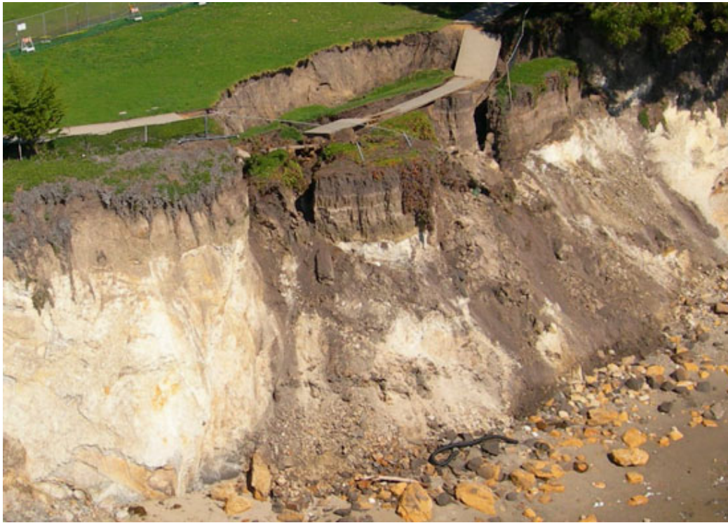
Figure 2.17 In January 2008, a landslide at Shoreline Park moved the cliff edge inland by as much as 12 meters (39 feet) and eliminated a portion of the sidewalk.
