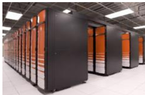
Figure 18: Data Center Using Advanced Cooling Controls
