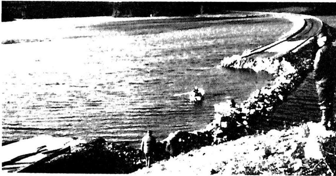
Fig. 1 View of the failure, October 4th 1983.
