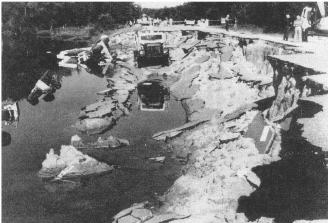
Figure A.9.2: Photograph showing the failed embankment (looking towards the west), showing crest loss and the positions of four of the large geophysical exploration trucks. (Hryciw et al., 1990).
