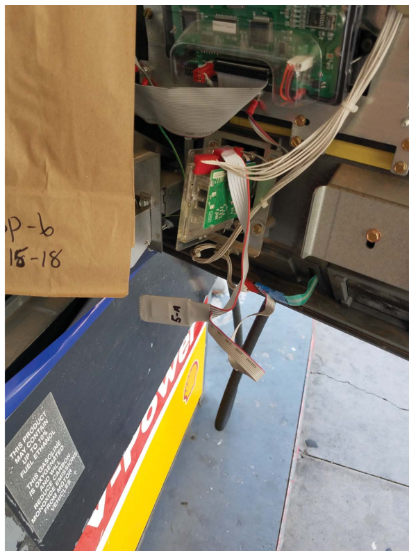
Figure 1.1: A skimmer taped the same color as the ribbon wire it is attached to.
