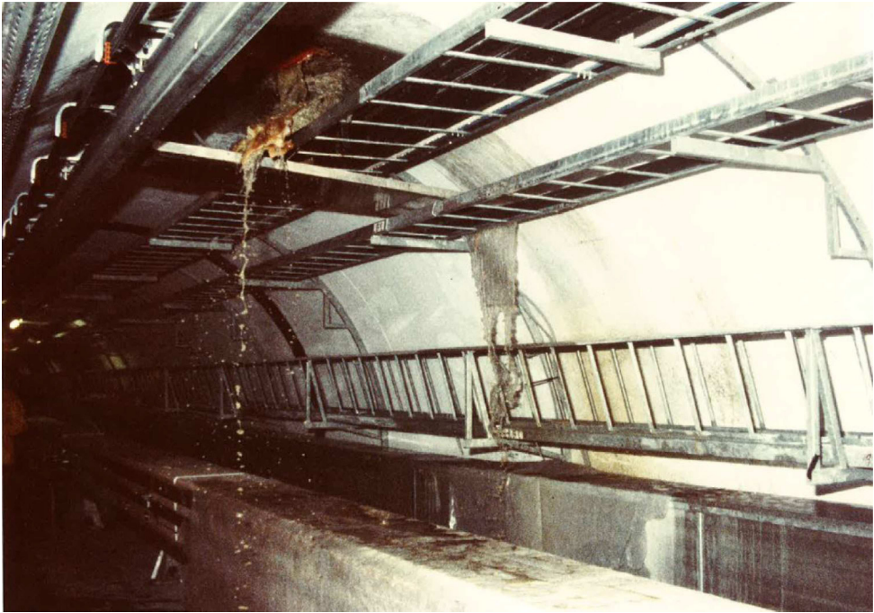
Fig. 4.11. Failure of tunnel concrete lining in 1990.
