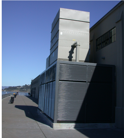
Figure 7.7 Cooling tower Pier 1 (Integral Group 2007).
