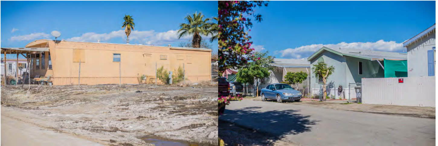
Polanco mobile home in Mecca, flooding can be observed surrounding the home
