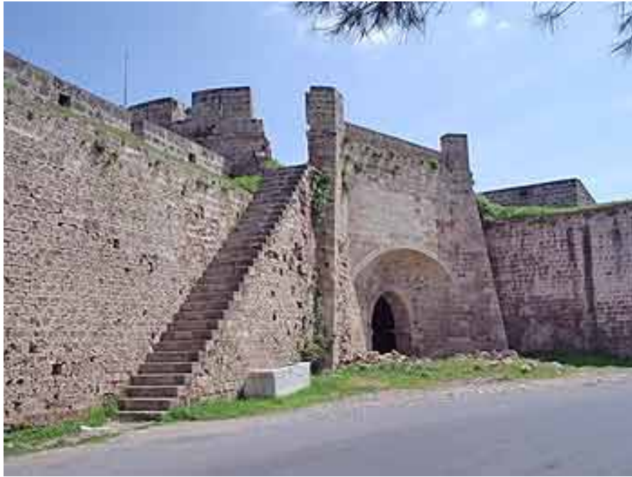
Figure 110. Stairs on city walls of Famagusta, North Cyprus, 2012. Photograph by Peter K.Lloyd / Alamy Stock Photo. http://www.alamy.com/stock-photo-famagusta-north-cyprus-staircase-up-medieval-venetian-city-wall-50977218.html , accessed December, 2017.
