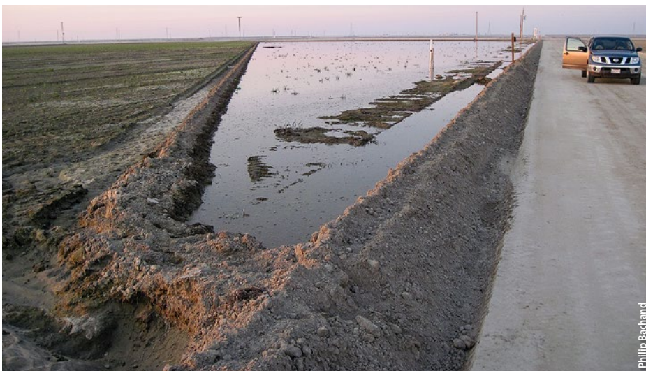
Wintertime modifications to tomato field to manage water were similar to rice checks to enable capture and infiltration of flood flows. Modifications included cutting small check berms to accommodate field gradients and installing low cost flashboard risers to manage water flow and elevations.
