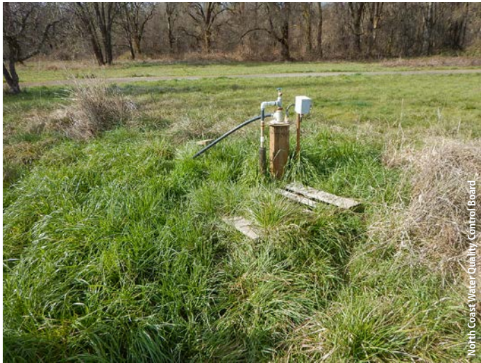
Subsurface water well. Well casing with associated power box and piping, used to convey water to storage or used for direct application.
