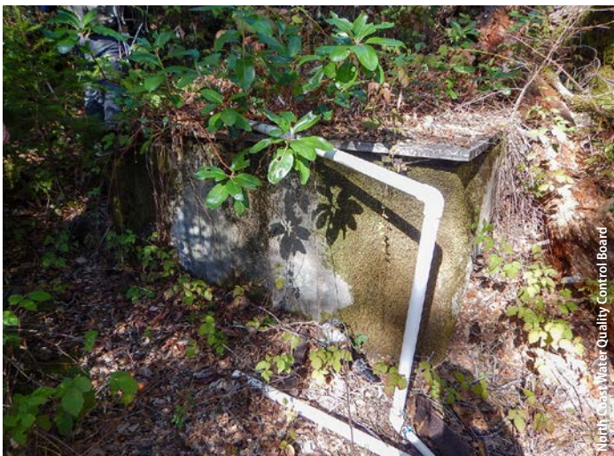
Spring diversion. Spring box installed to consolidate flow, which is then directed through PVC piping.
